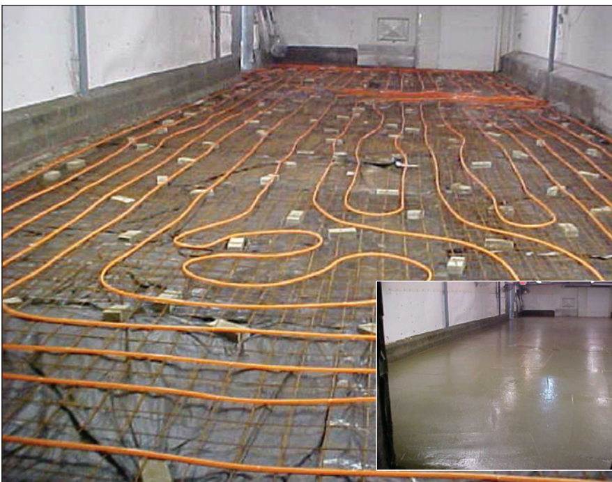
After removing the damaged concrete floor, the contractor's crew placed the heated tube system (above) and installed a new, four-inch concrete floor over the tubing (inset).
